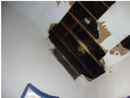
Image 09- SW Sanctuary Roof Leak
