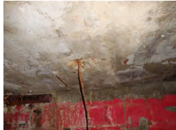
Image 16- Slab underside damage
