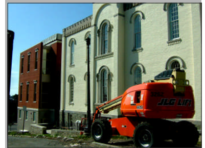
Rehabilitation of the Oswego Library was partially funded through the Environmental Protection Fund. The Section 14.09 review considered the addition's distinct, yet compatible design.
